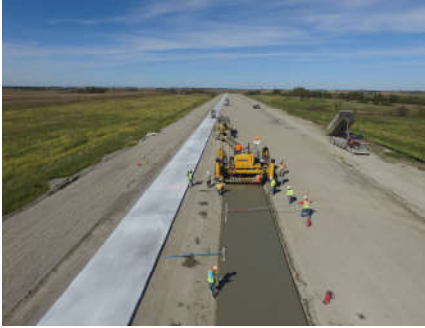
Reliever & General Aviation Airports Runway 14/32, Taxiway & Apron Reconstruction at NW Missouri Regional Airport
